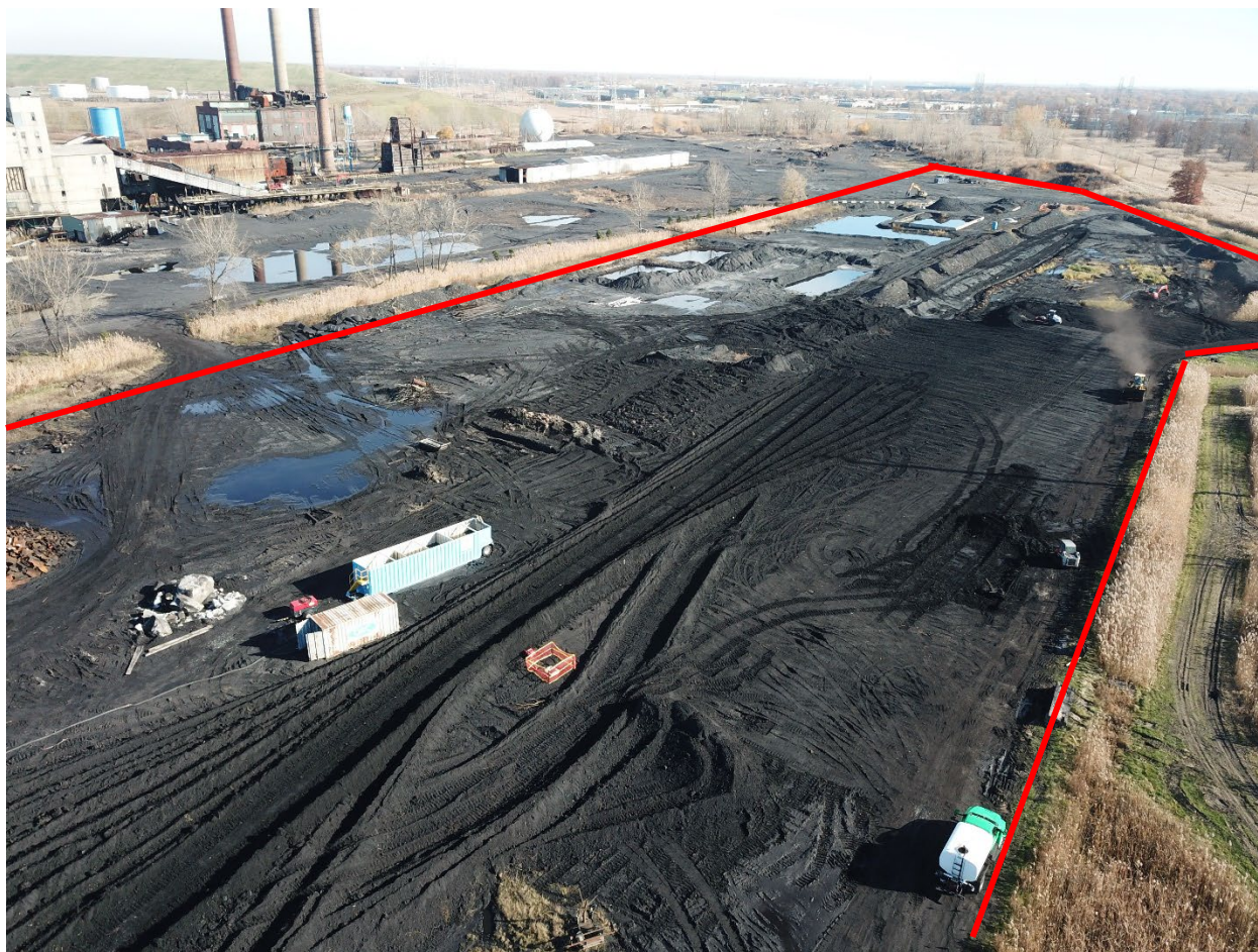
Photo 4-8: Looking Northeast across the Coal Yards during regrading and prior to establishing stormwater BMPs.
